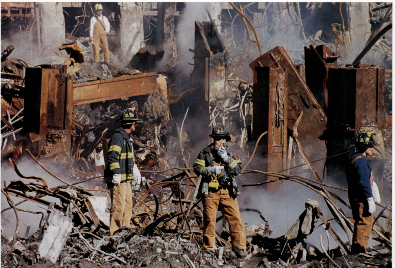
Figure 3-5 The core column in the center appears cut by a torch. The workers cut the steel so quickly that it is difficult to determine which damage was from them.
