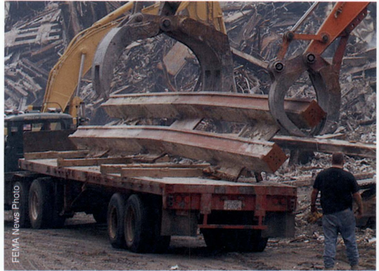
Figure 3-10 Two columns still attached to the three plates that made a pre-fab unit.
