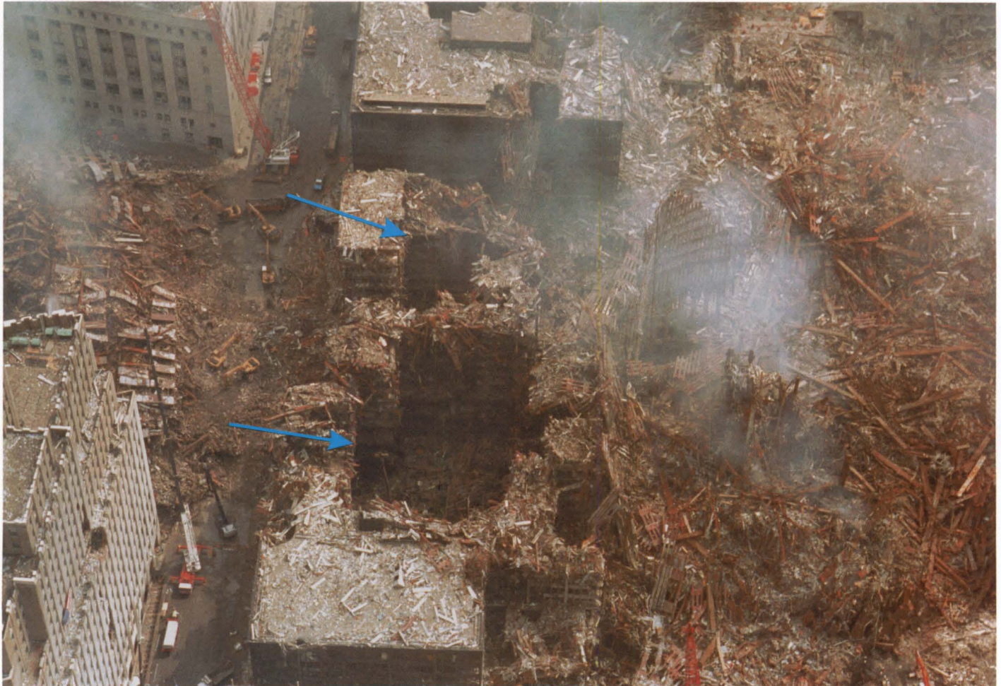
Figure 1-2 The blue arrows point to two deep holes in Building 6. Did falling debris create those holes? Or were those holes blown open to release the high pressure in the basement?
